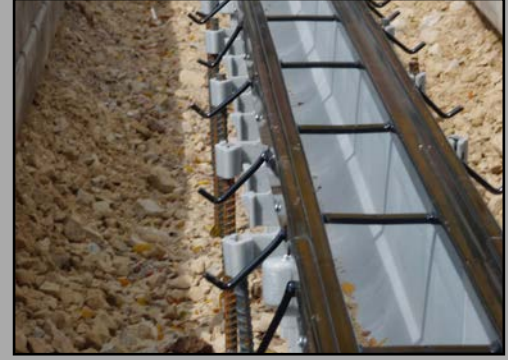
Storm water inlet repair and installation, pipe work, sub-surface drains, trench drains
